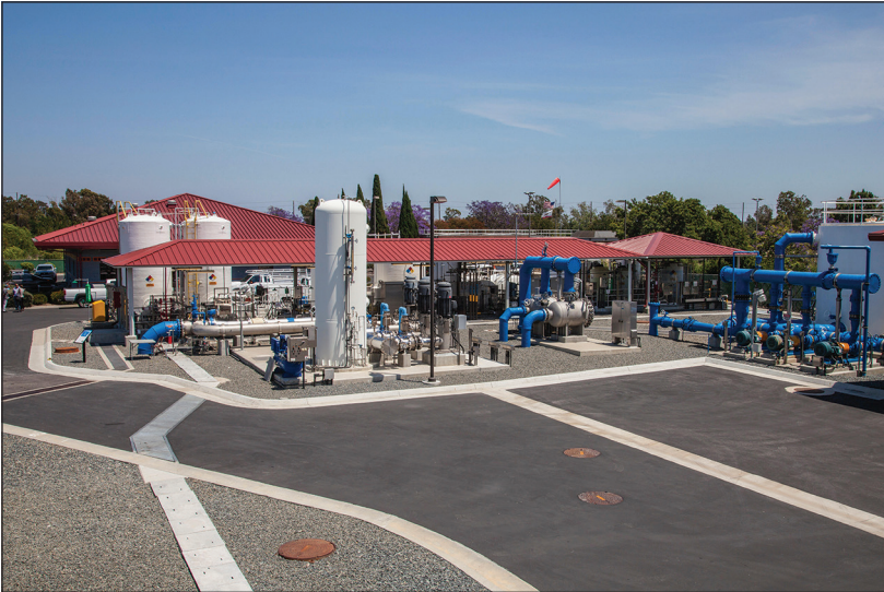
A pumping station near Perth abstracting water from underground stores
